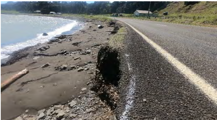
Figure 10.5: Undermining of SH35 within cell 10A
