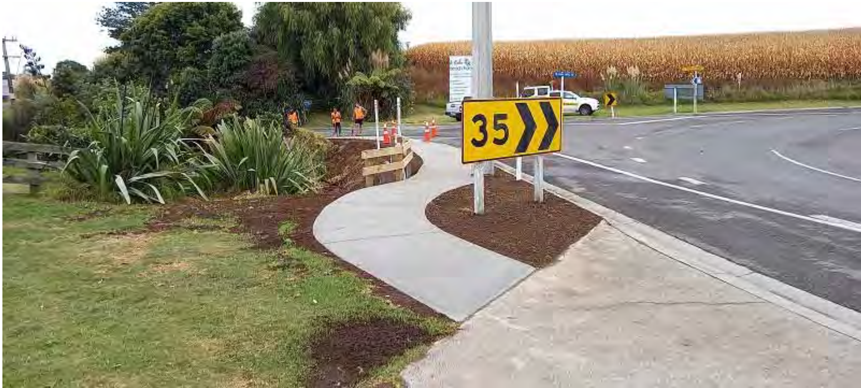
Footpath installation in Te Kaha with funding provided through the Provincial Growth Fund
