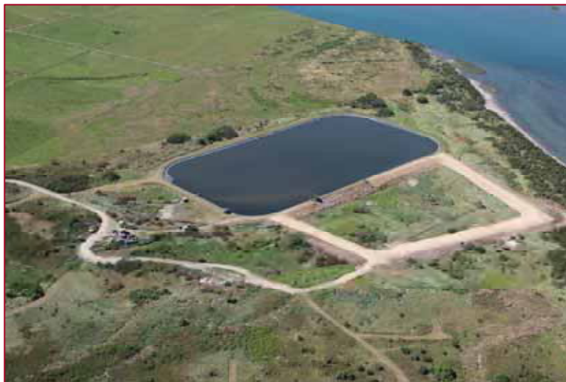
Image: Ōpōtiki Sewage Treatment Pond showing extension
