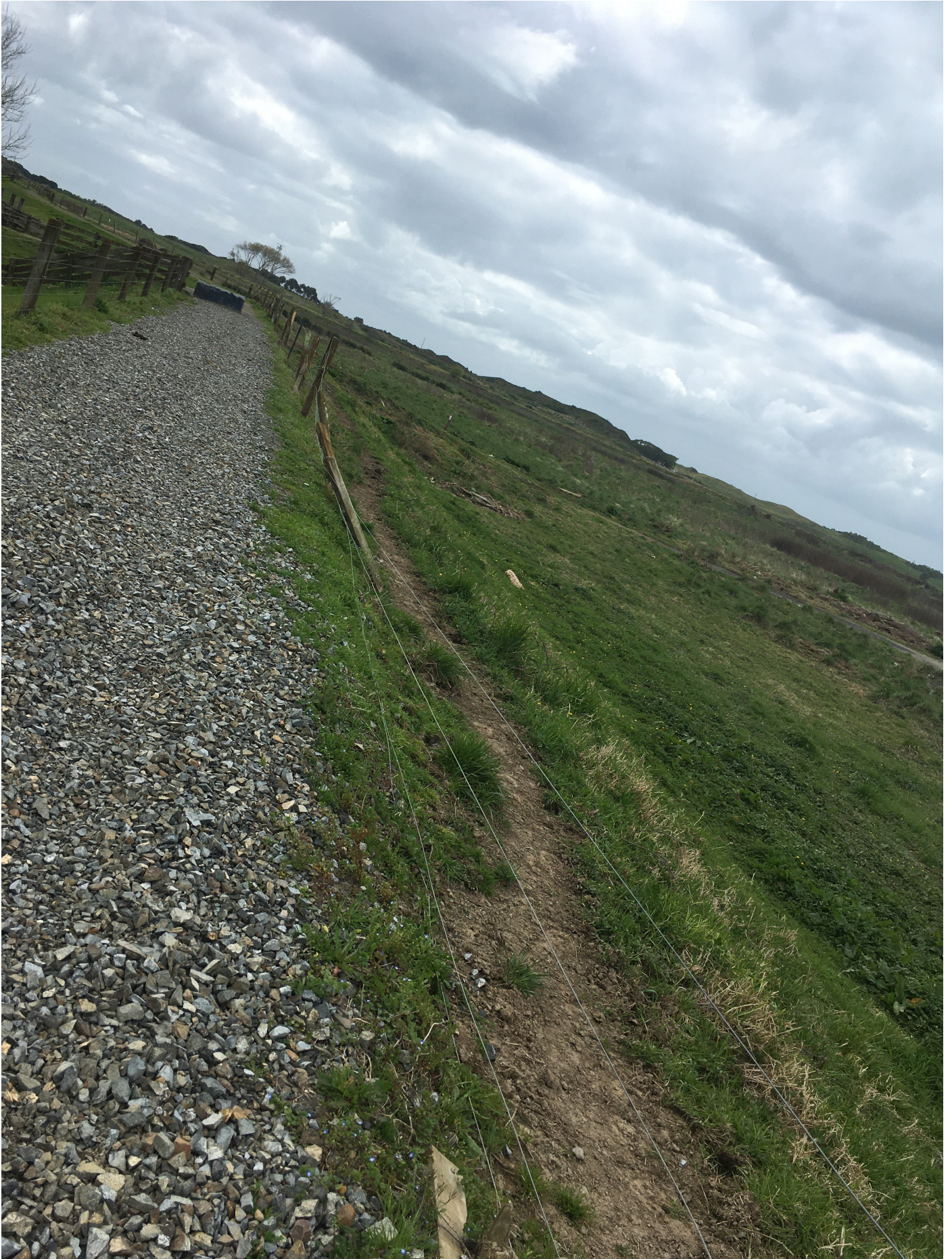
Another shot of the damaged wire and posts and stop bank near the pony club next to the Otara River. 22/9/21
