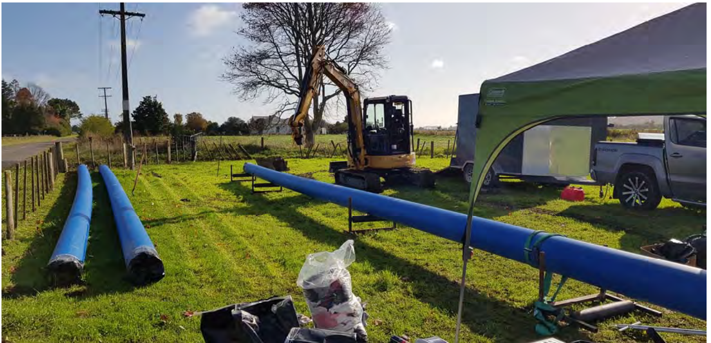
Image: Welding of pipes to replace the ageing raw water supply main along Otara Road from Clarks Cross Road to the pump station is in progress.
