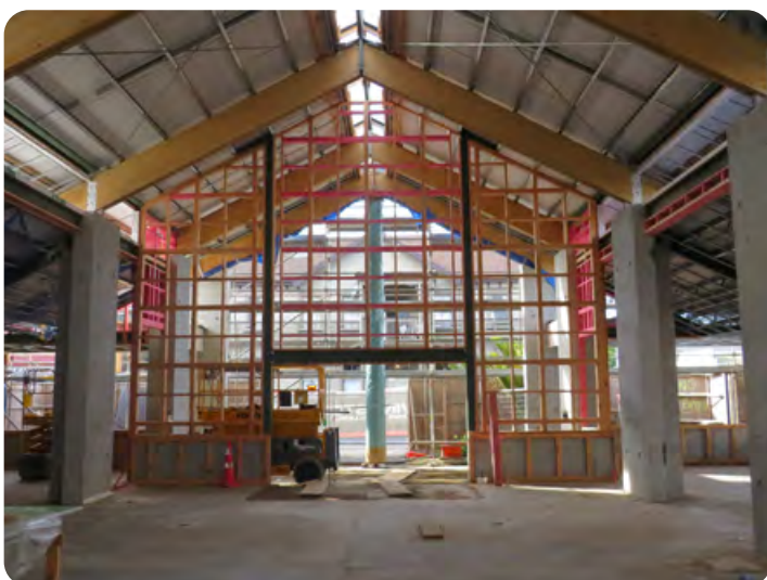
Te Tāhuhu o Te Rangī is progressing well and on track for a formal opening in October. This incredible building will provide the same services as currently offered through our Library and Digital Hub and a wide range of new opportunities including meetings rooms, holiday programmes, new resources and social spaces.
