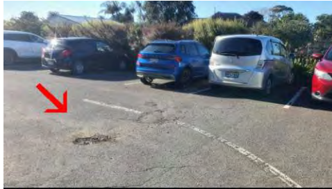
Repairs required to driveway
