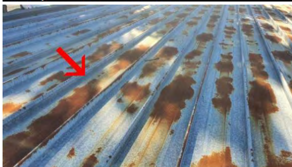
Heavy rust noted
