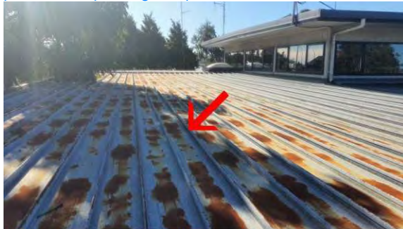
Widespread surface rust noted
