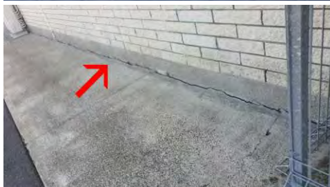
Cracking to plaster hunching noted
