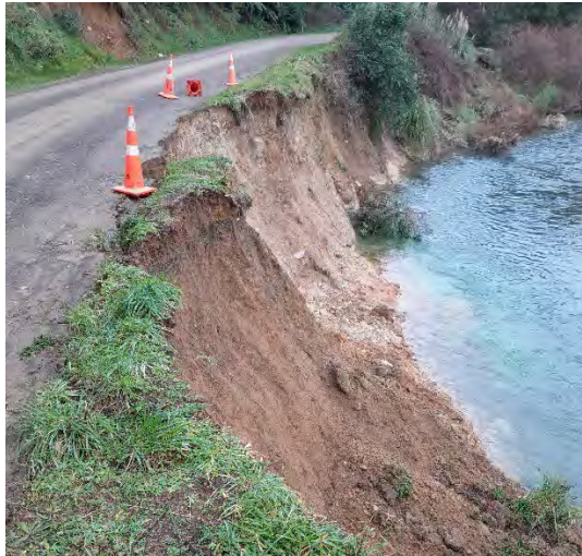
Figure 3: Washout on Waitahe Valley Rd – ODC (18/07/2022)
