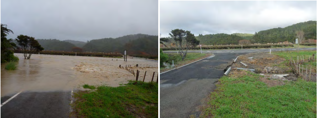
Figure 2: Flooding and subsequent road damage - Ngarue Rd, Whangaparaoa. – Provided (13/07/2022)
