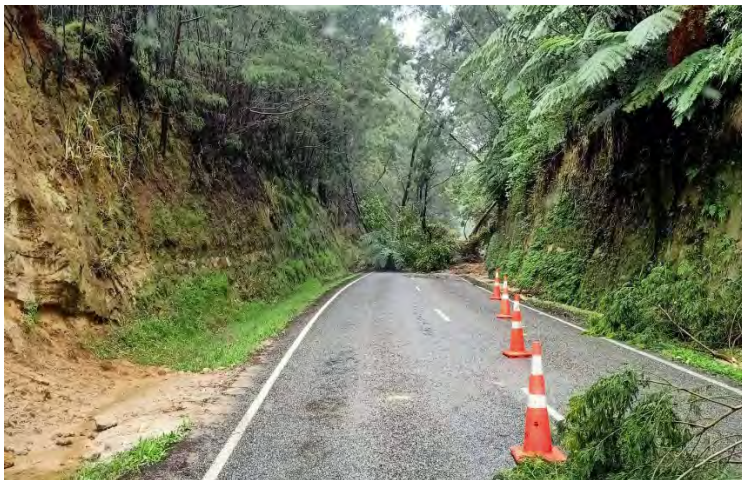
Figure 7: Treefall and road closure on Ruatuna Rd
