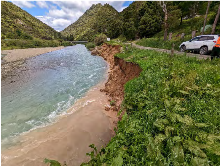
Figure 6: Washout alongside Otara Road
