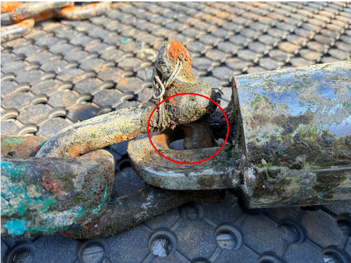
Picture showing wear on the pin of the shackle
