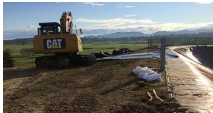
Step 1 – Tidy up around the reservoir (the pine needles created constant maintenance issues so the trees were felled and this area will now be grassed for easy maintenance).
