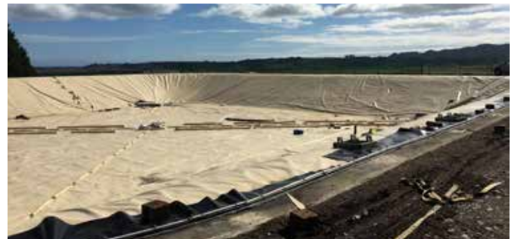
Step 5 - Re-fill the reservoir then sterilise (hyperchlorinate) and flush. Re-sterilise with low dosage chlorine and test. Repeat until all clear before reconnecting to the town's reticulation. For the final image showing what the town's reservoir looks like now, check out our Facebook page
