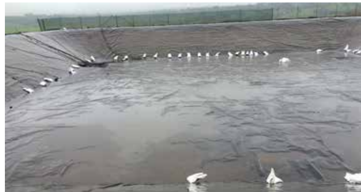
Step 3 – Check, minor maintenance and clean the dam liner while the reservoir is empty.
