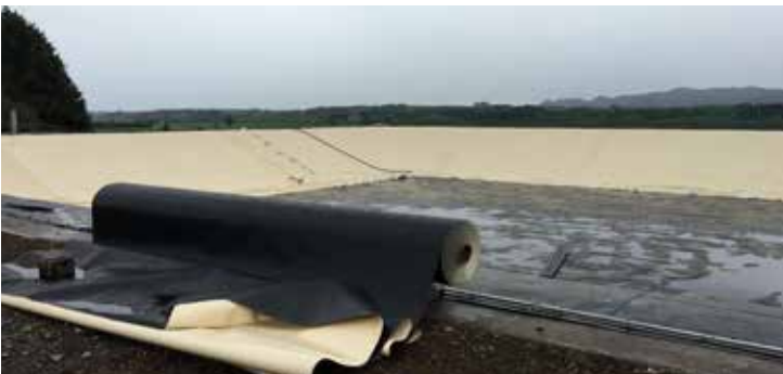
Step 4 – Lay out the new lid in sections on to the empty reservoir and install weights on each of the diagonals to prevent the cover lifting in high winds. The original poles and weights system is no longer needed. Join and fix the cover together so that it is completely sealed.
