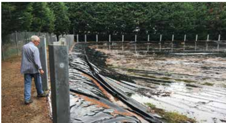
Before photo – The old reservoir cover had cables, posts and weights to ensure it didn't lift in the wind. There were signs of wear and a risk that stormwater could contaminate the reservoir.
